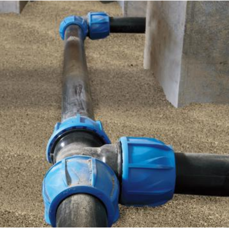
Water Distribution Lines
